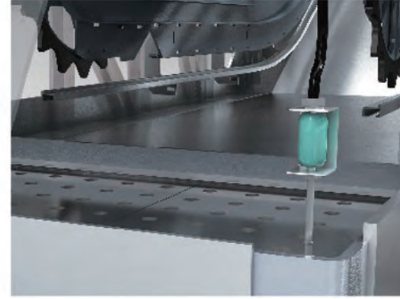
Lower machine room installation water level detection sensor(ladder outdoor)
